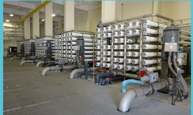
Pompano Beach Full Scale NF Plant
