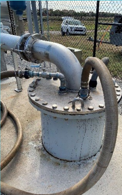
Wellhead with Acid Injection Line
