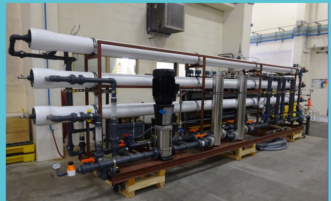
Pompano Beach NF Pilot Unit
