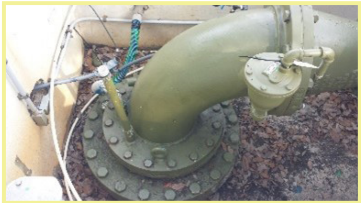
Original Well 6 Wellhead
