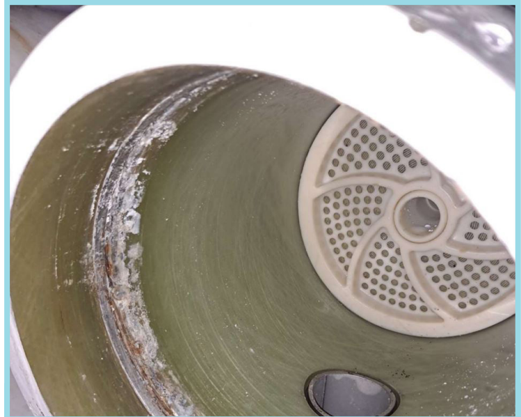
Figure 3. Corrosion of Bearing Plate onto Shell
