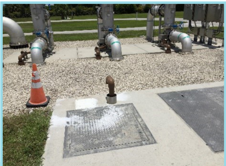
Modified Sand Strainer Drain Lines
