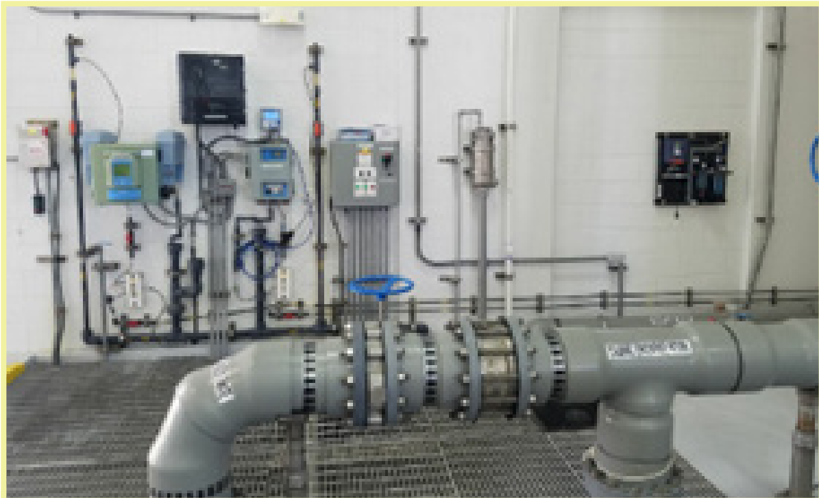
Four-log Treatment Monitoring Equipment: Chlorine & Ammonia Analyzers
