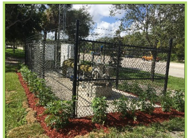
Replacement Well #4R
