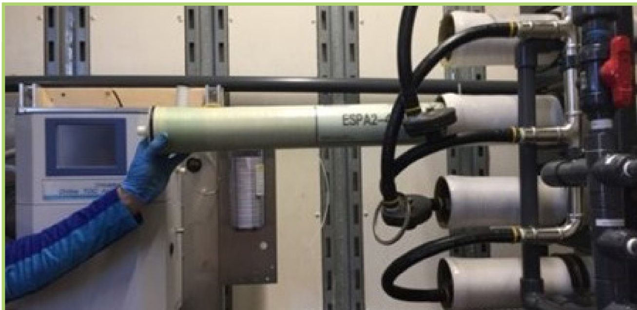
Figure 10. During startup of the RO system, new reverse osmosis elements were installed, as well as an in-line TOC analyzer. In-line TOC analyzers are not widely-used, and this innovative instrument helped operators monitor treatment performance in real time.
