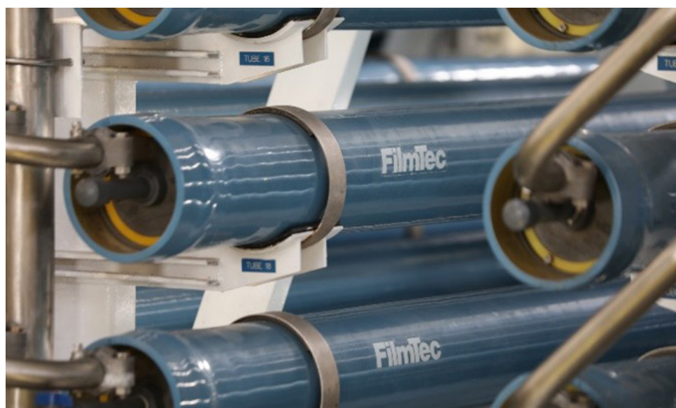
Image 3: Close up of RO modules
