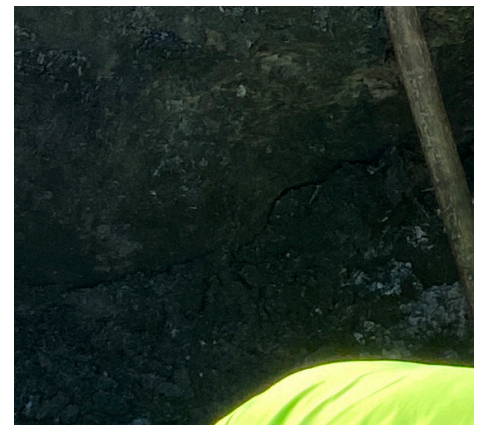
Lead Service Replacement Header
