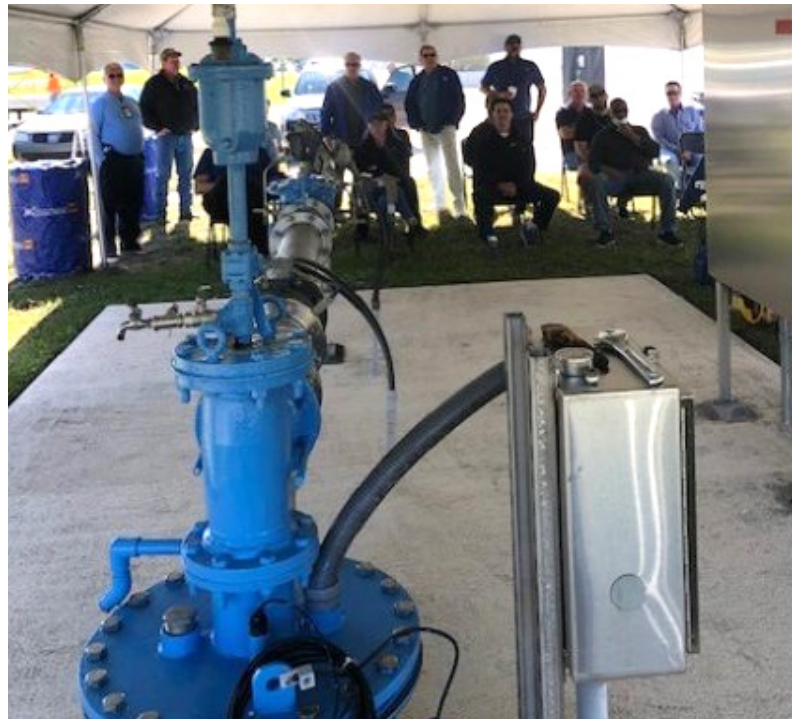
Well #3, Wellington Water Plant
