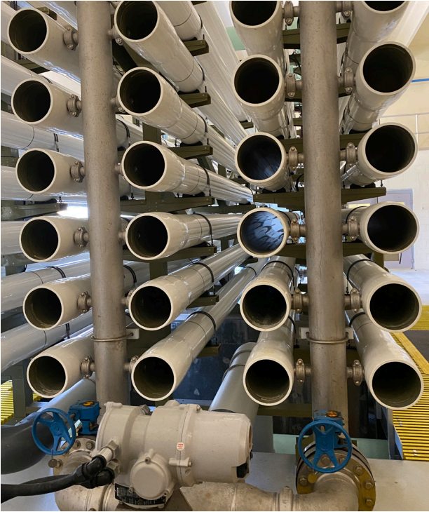
Train Unloading of Old Membranes Elements
